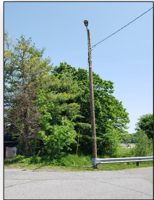
New light pole.
