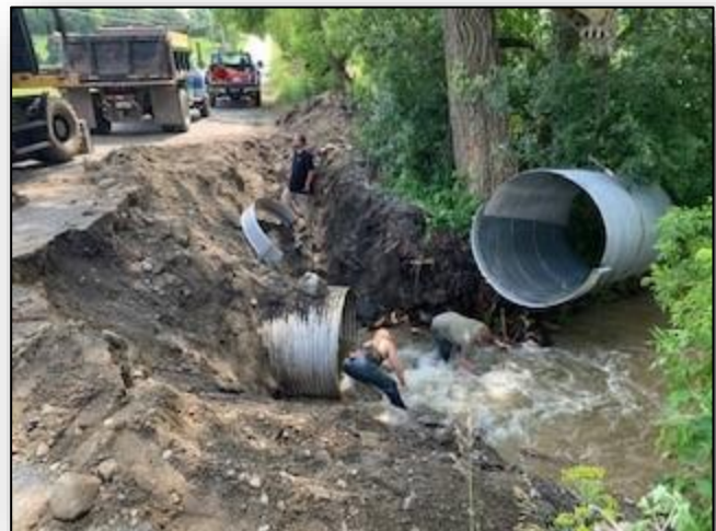
FEMA reimbursed projects like this washout.
